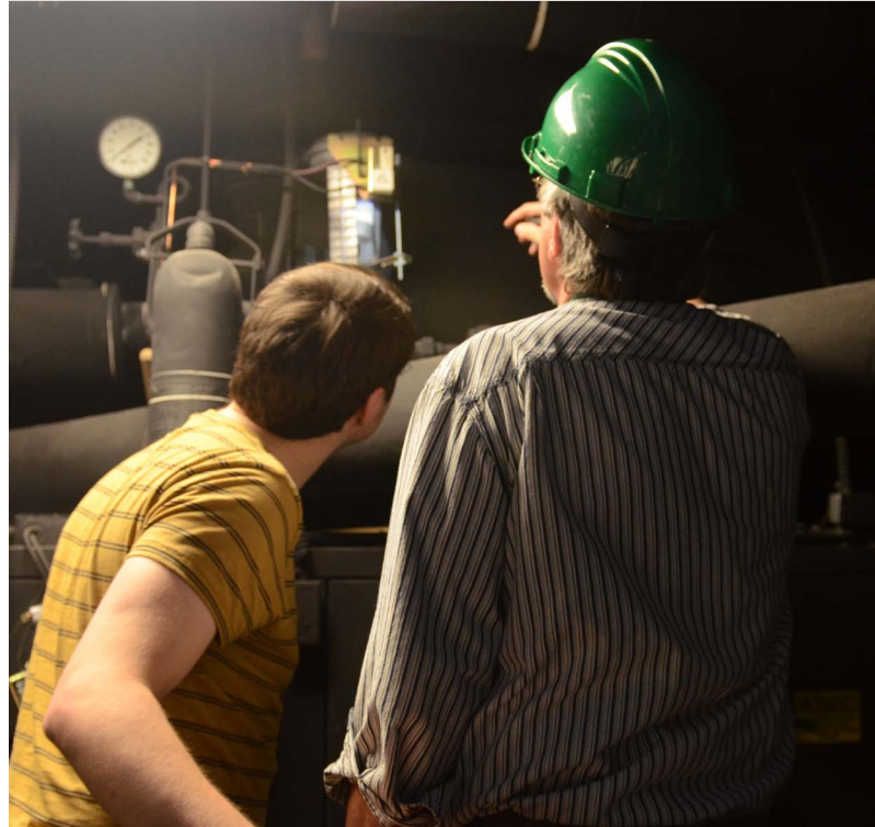
Michigan State University facilities employees observe a gauge in a boiler room while participating in a Spartan Treasure Hunt.
