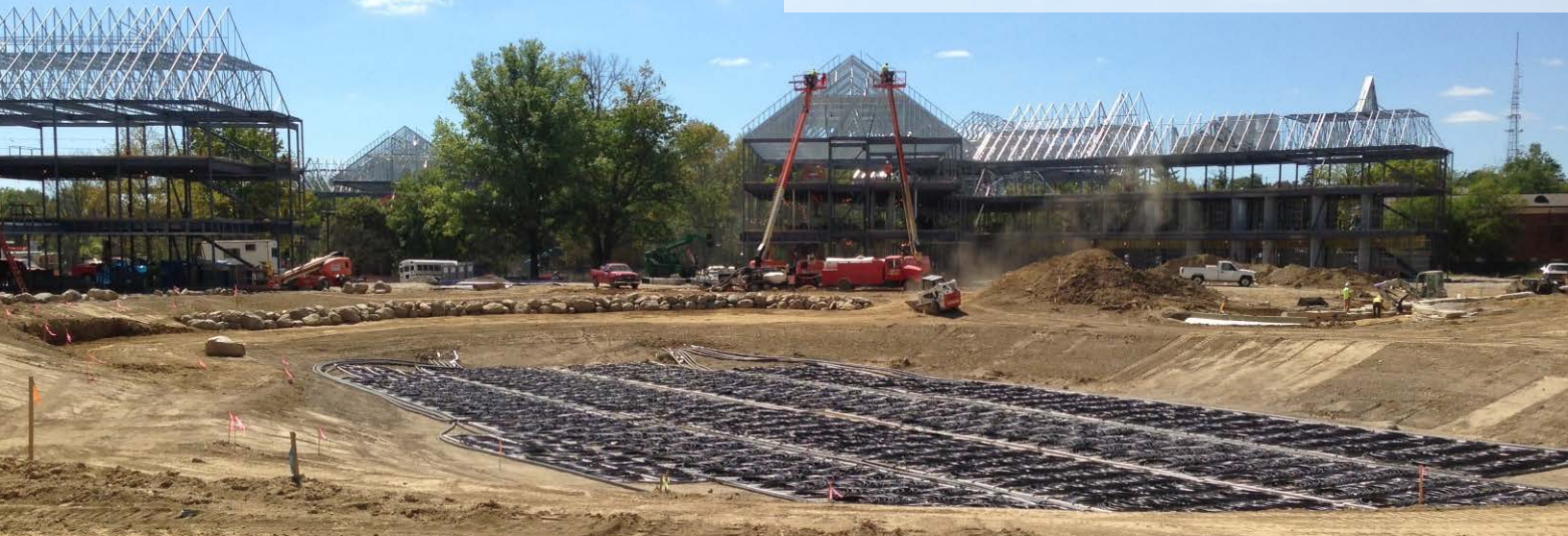
Installation of coiled heat exchangers in the upper pond at Miami University (top) and after completion (bottom).
